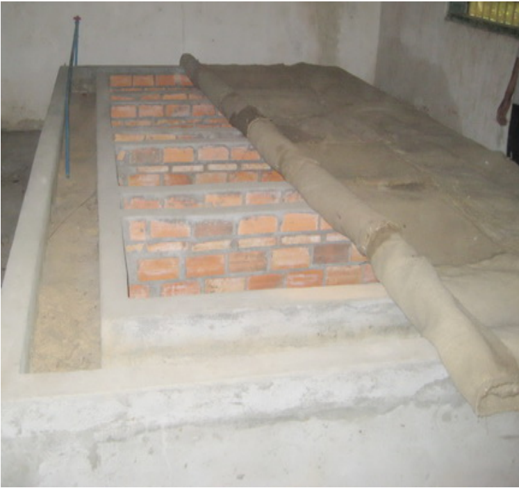
Brick-walled EC 4.5x2.5x0.6 m in length, width & height, 15-20 cm double wall with moist sand
